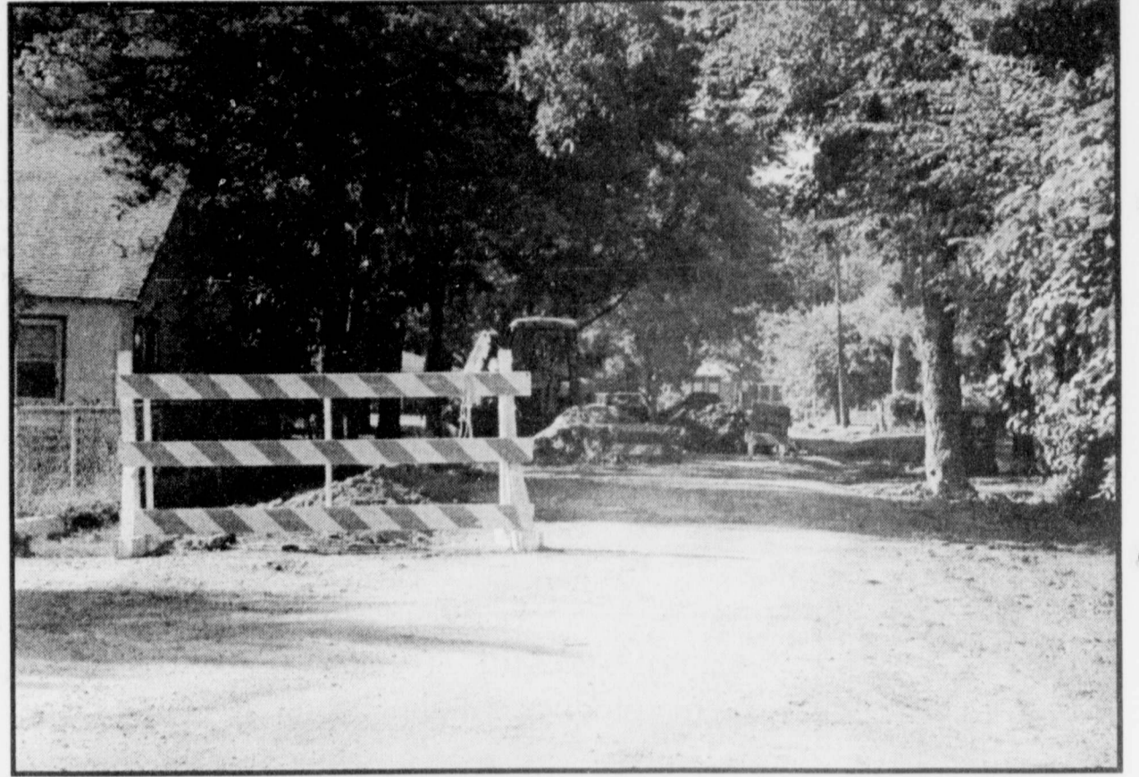
CONTINUED WORK-work continues on the new sewer line in Deport on College Street. After the sewer line is installed the road will be fixed. (Staff Photo by Nanalee Nichols)
