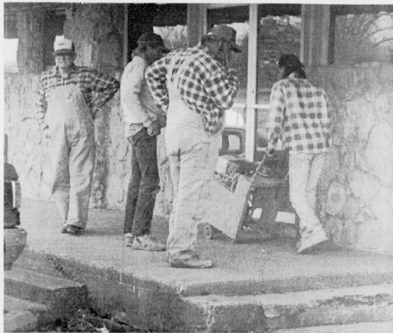
LOOKING ON-Deport Mayor Charles Foster and Construction Superintendent Dale Young look on as workmen from Payne Construction prepare Handicapped Ramps in Deport last week. The work is funded by a federal grant and the city will not have to absorb any of the cost. The handicapped ramp makes downtown Deport accessible to those with disabilities for the first time in many, many years. Deport's sidewalks are unusually high, because they were built many years ago when Main Street would flood. (Staff Photo by Thomas Nichols)
