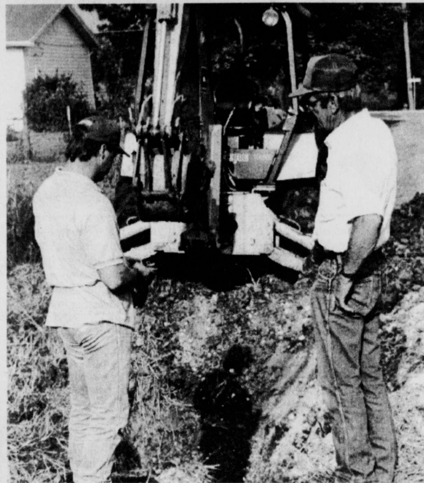
MISSILE! -instead of digging up the road surface in Deport this week, the City of Deport had a machine come in which forces a "missile" under the road surface. This means that a new water line can be run under the street with no damage to the surface. City Water and Sewer Superintendent looks the situation over with the operator of the machine. (Staff Photo by Nanalee Nichols)
