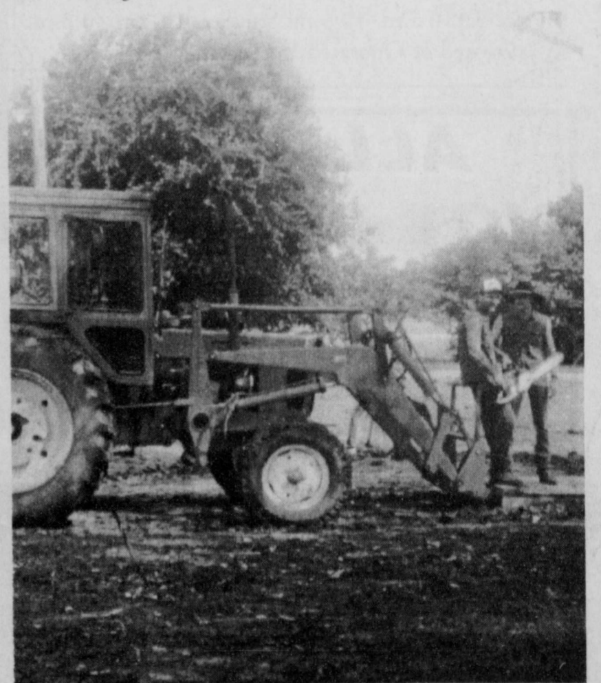
SETTING POLES -David Shelton (in tractor), Steve Richard and Thomas Crossland put up poles for a volleyball net at the location where the old community center was located.
