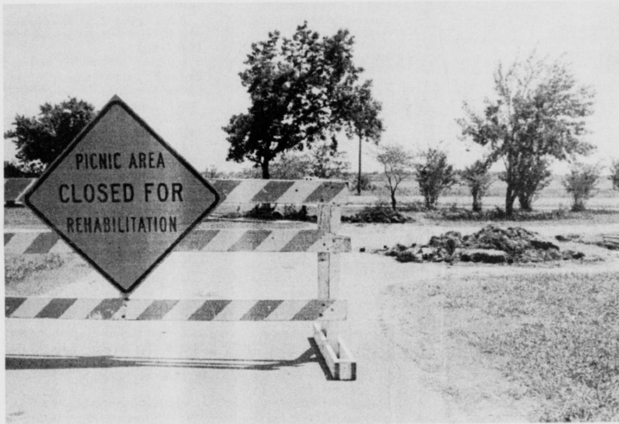
TEMPORARILY CLOSED-the park at the west side of Deport is closed for rehabilitation right now as the Texas Department of Transportation pours handicapped access facilities and trims trees and gives the park a "facelift". (Staff Photo by Thomas Nichols)
