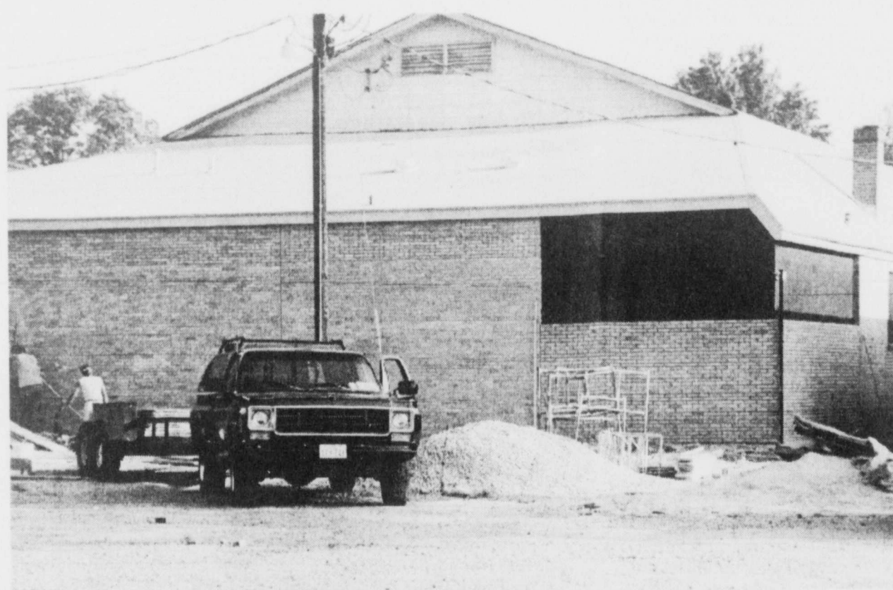
NEW ADDITION-A science lab that meets all state standards and full dressing rooms for boys and girls is under construction and nearing completion at Deport Junior High School. The brick work and style has been matched to the existing structure. In addition, a metal roof is being put on the two story grade school building, which has had a leakage problem for many years. (Staff Photo by Nanalee Nichols)
