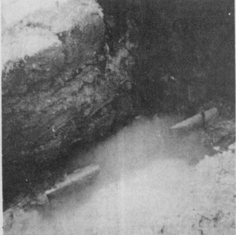
LARGE HOLE-this huge hole is the result of a six inch sewer line rupturing in Deport 4-30. The line was at the north east corner of the Full Gospel House of Prayer Parsonage. City Officials and Hayter Engineering
