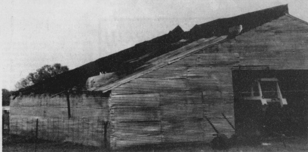
HEAVY DAMAGE -This barn belonging to Charles and Cindy Nichols of Deport suffered heavy damage during last Wednesday's storm. The barn was full
