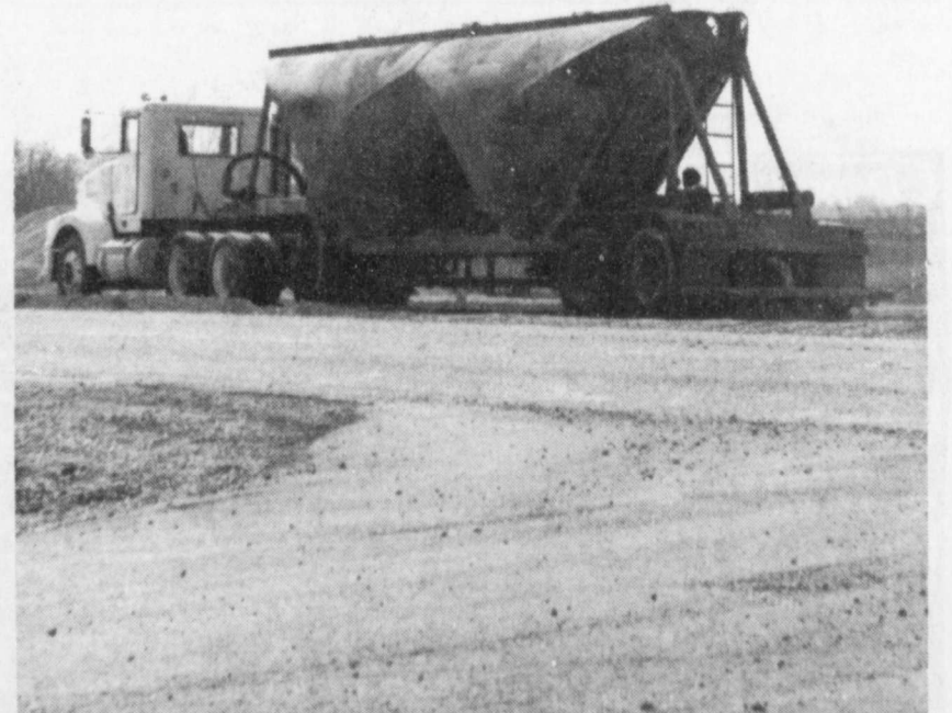
PROGRESS- Huge cement trucks were busy leaving cement to be worked into the gravel on
