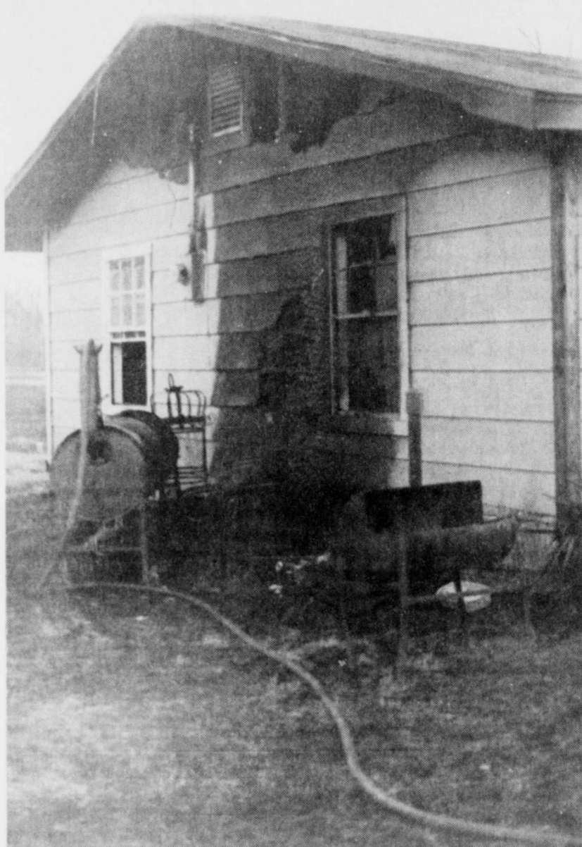
DAMAGED-Ricky Fox's home in Cunningham was damaged by fire when a grass fire caught a stack of tires next to his home
