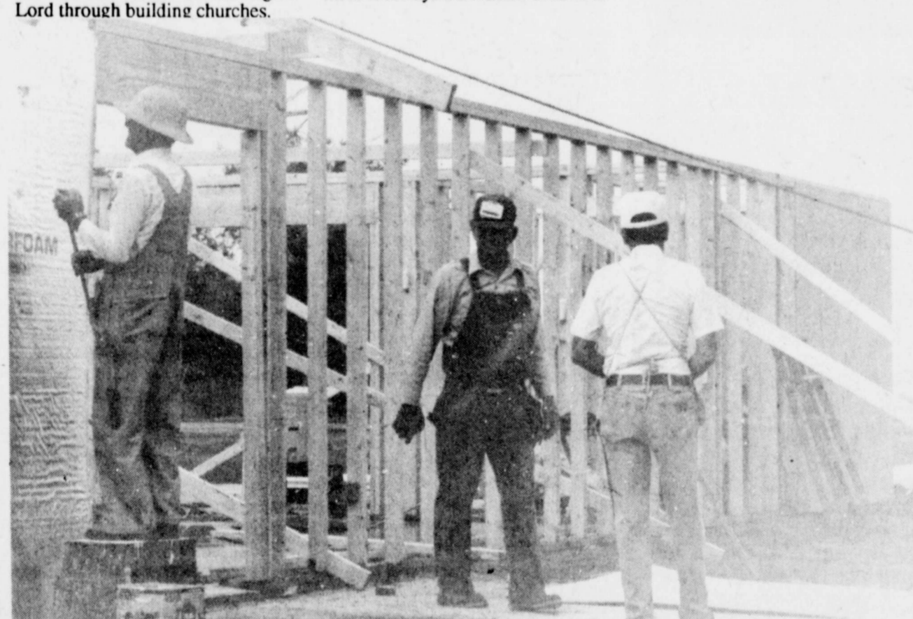
GOING UP-Twenty three retired Baptist men were on hand Monday morning to begin building the Cunningham Baptist Church. The group travels all
