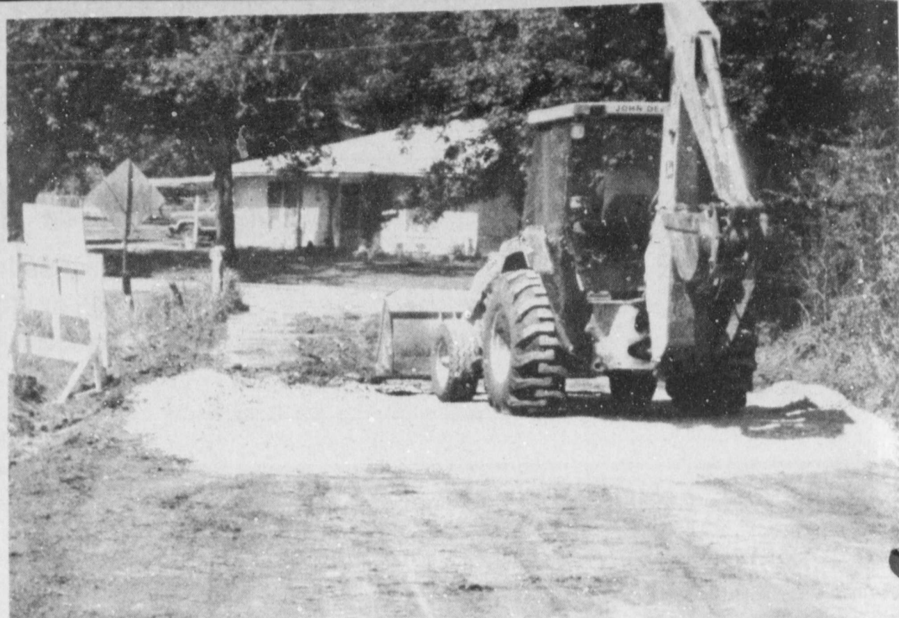
BUSTER PAVING Co. of Sulphur Springs has been working on Jeffus Street in Deport
