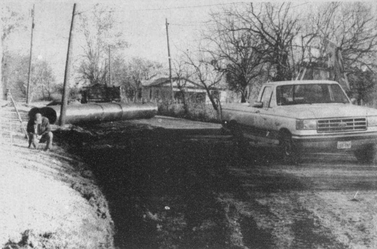
WORKERS from Spann Construction Company of Mt. Pleasant have been busy preparing portions of Depot and Nobles
