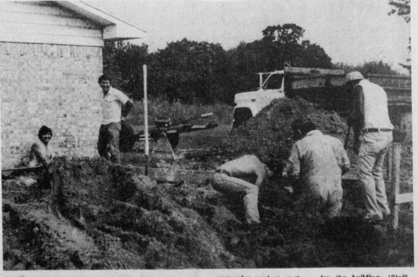
NEW ADDITION- Legion Post, preparing the ground for pouring a foundation for the new expansion project at the post. The new addition will provide more area for the building. (Staff Photo)
