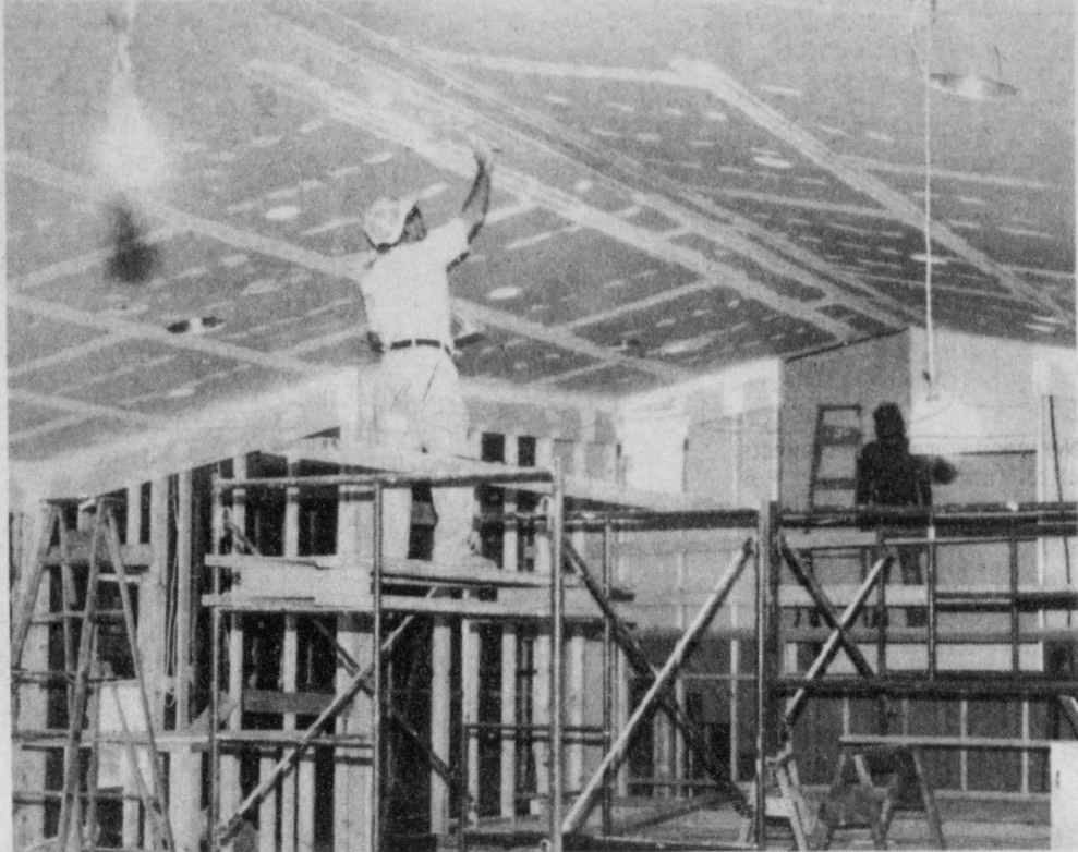
INTERIOR WORK—the new Faith Baptist Church is nearly complete. Sheet rocking the ceiling, and installation of carpet and other finishing touches are foremost on the minds of workmen and the congregation. (Staff Photo)
