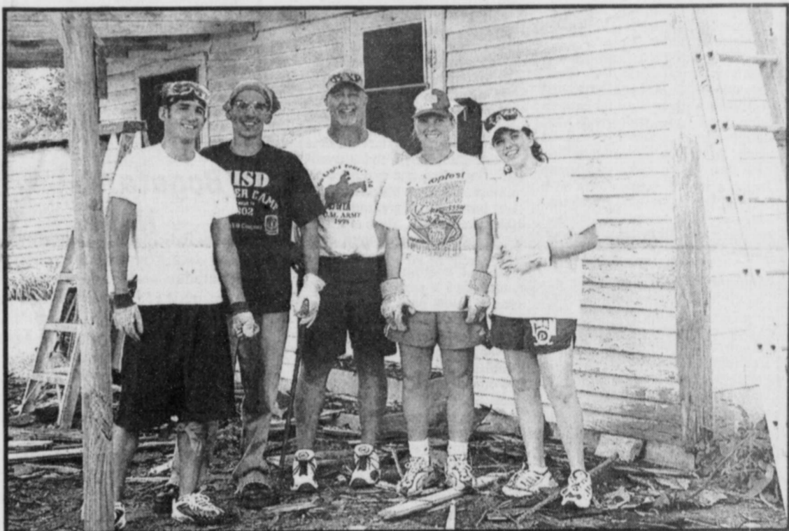
UMA-the United Methodist Army is in town this week making repairs to homes belonging to those who are unable to make repairs themselves. The group pictured are from Houston and were working on the home of Chrystine Baker, repairing the carport and trim. The youth's sponsor said the group had cleaned out a huge amount of wasp nests and were surprised the insects had not attacked anyone entering the house from the carport. Other groups are working on several homes in Bogata and will make repairs to up to 15 homes before leaving. (Staff Photo Nancy Brown)
