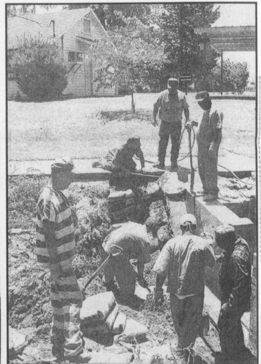
BUILDING A NEW DAM -Juan and Ted Torres in the background assist inmates from Red River County jail build a new dam across Morrison Creek in Thomas Park last week. The spring fed creek will be bank full this Saturday for the annual duck race during Frontier Days. The Torres donated their time and expertise to build the new dam.
