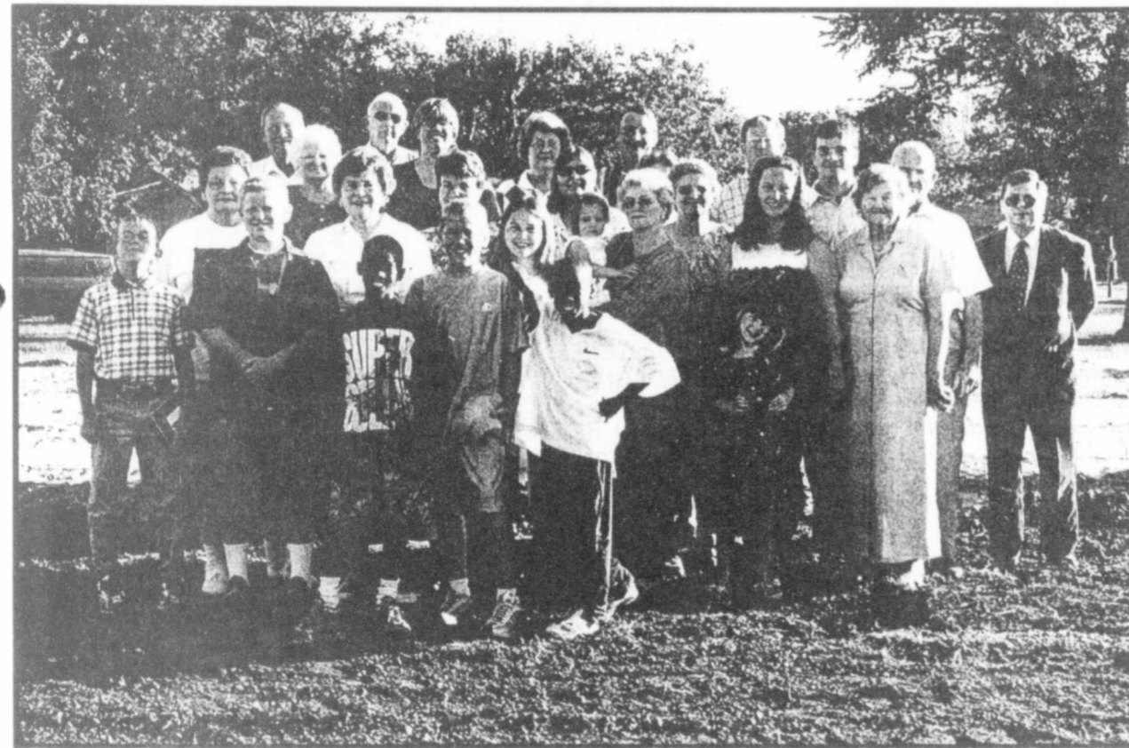
GROUND BREAKING-The Talco Church of Christ congregation is proud to announce the beginning of a new church parsonage located directly across from the church in Talco. The foundation work has begun and Pastor and family, Bryan, Melinda, Jasmine, Jasper and Chloe Hodge can't wait to move in. (Staff Photo Nancy Brown)
