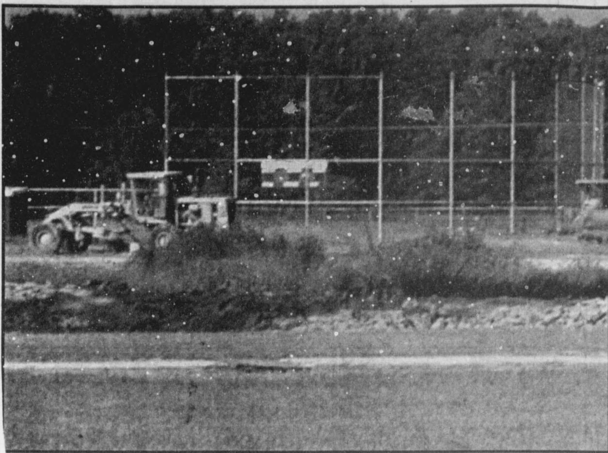
CLEAN UP-Wright Excavating had equipment at Rivercrest High School this week doing clean up work between the back of the school and the boys baseball field. The old sewer ponds were filled in and the extra space will provide more room for activities at the school. (Staff Photo Nancy Brown)
