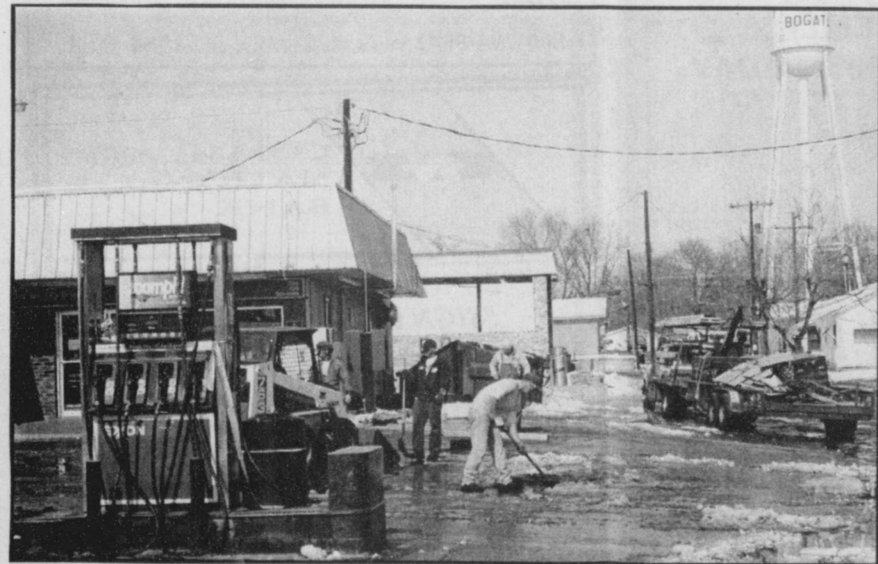
CLEAN UP CONTINUED-at the Armadillo Kwik Korner in Bogata on Sunday after the snow and ice caved in the awing over the gas pumps at the store. The store was open for business on Monday. (Staff Photo Nancy Brown)
