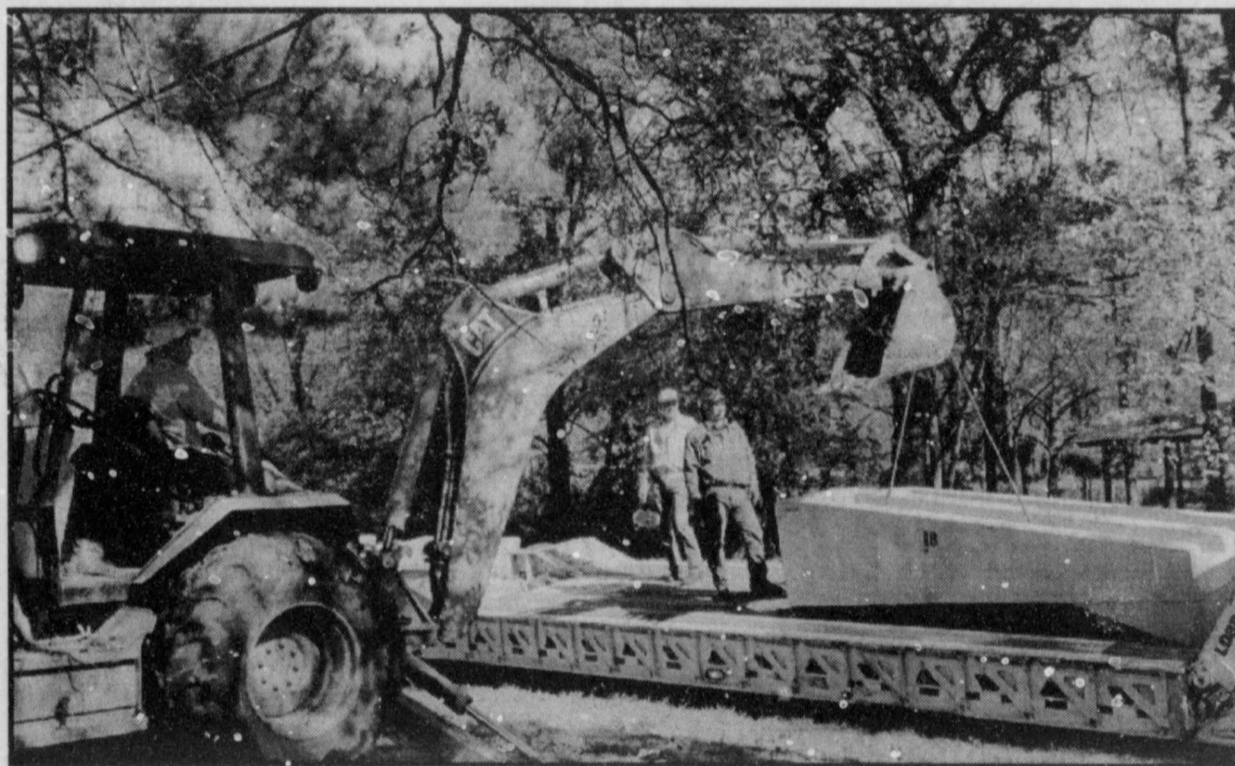
WORKERS with Paul Drake Construction Co. of Powderly have been busy this week preparing the site for St. Joseph's Medical Clinic-Bogata. Being unloaded are culverts for the driveways leading into the new facility. The clinic is set to opening November 18th. (Staff Photo by Thomas Nichols)
