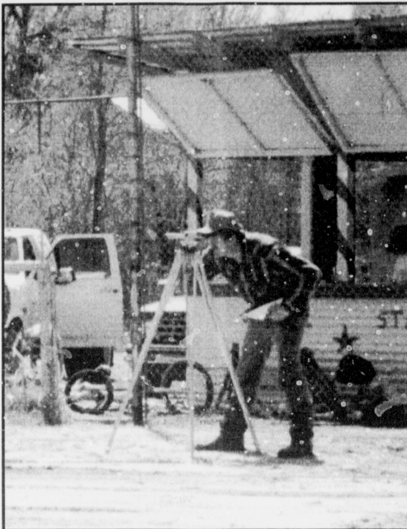
SHOOTING A GRADE -Randy Hollis checks the grade on the Talco ballfield at the work day held Saturday March 23. The group were able to get major dirt work done on the field, plus painting and welding work. Everyone who attended and helped by providing equipment and supplies were greatly appreciated. (Staff Photo Nancy Brown)
