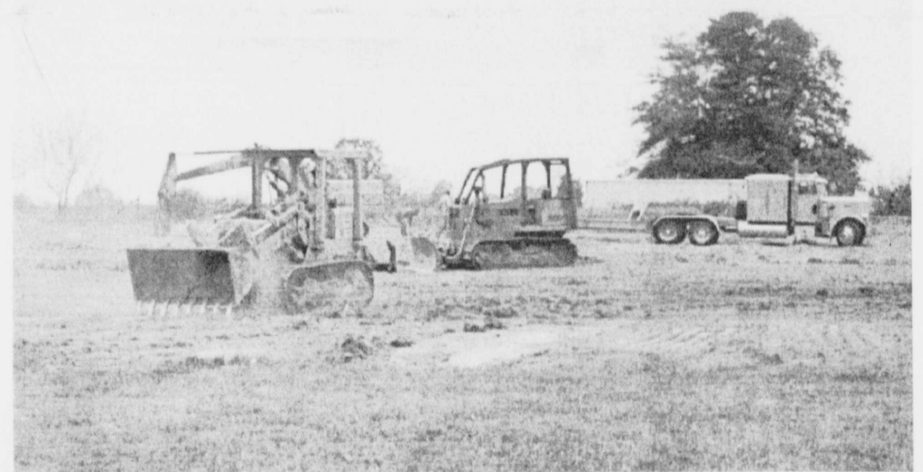
DIGGING UP THE DIRT- The dozers and backhoes arrived early Saturday morning to prepare the land for the new housing units to be built on Highway 271, in Bogata. The
