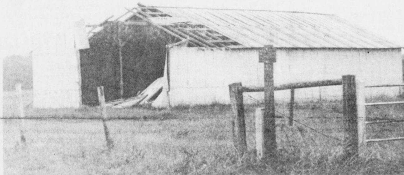
TORNADO DAMAGE-barns, trees, homes and vehicles suffered heavy damage through-
