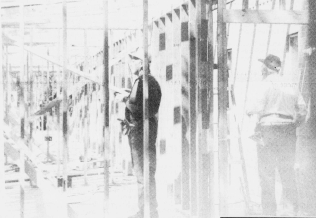
The Fulbright Baptist Church is building a fellowship hall onto the existing structure. The work is being done by contribution
