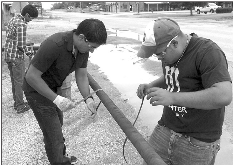
NEW GOAL POSTS —Rule juniors, Luis Diaz and Paul Nieto, work on new goal posts for the Rule football field. Students built the goal posts under the direction of Monty Moeller at the new Vocational Technical Center in Rochester, using pipe donated by Wilcox Oil Company in Rule.
