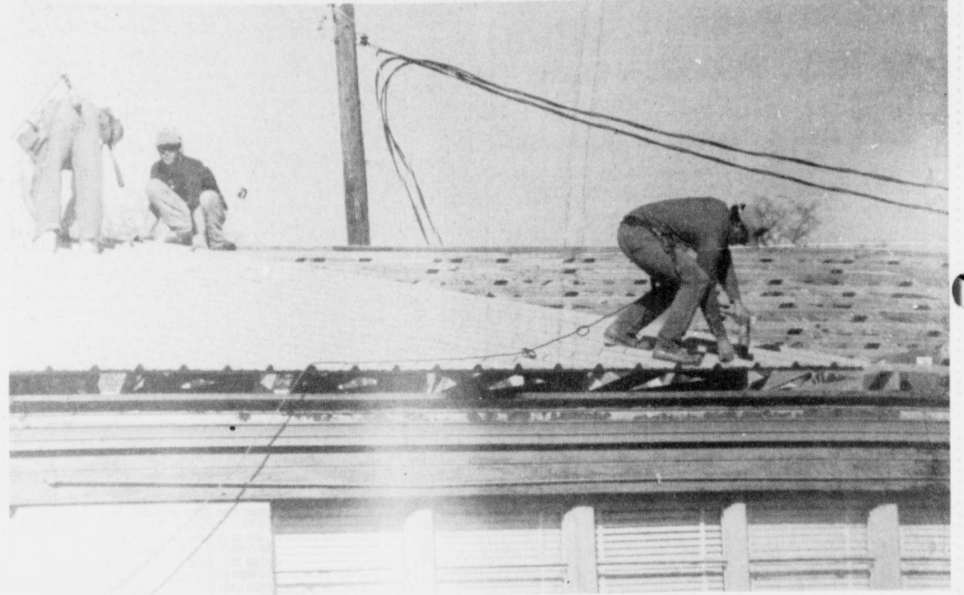
PARKER CONSTRUCTION Company of Pittsburg is busy re-roofing the Bogata Elementary School. (Staff Photo by Keye Lee)
