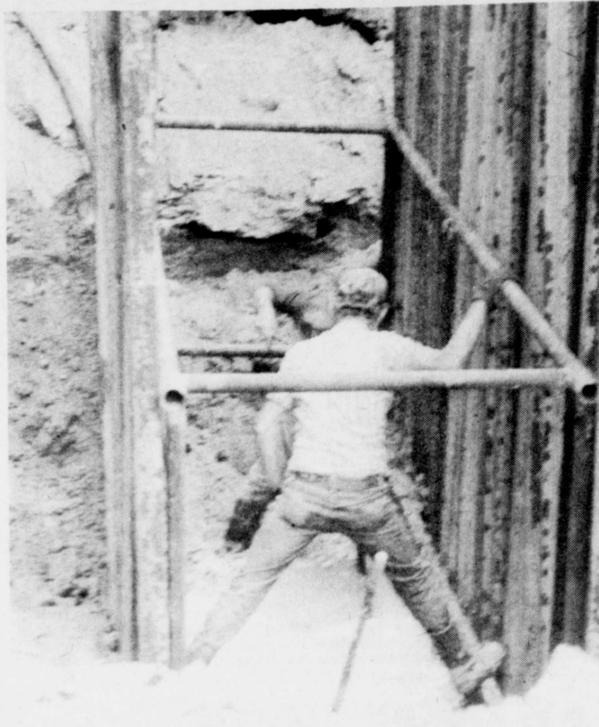
CITY EMPLOYEES of Bogata, Rick Cox and Hollis Moore, look for a broken sewer line to be repaired on 3rd NE Street Tues-
