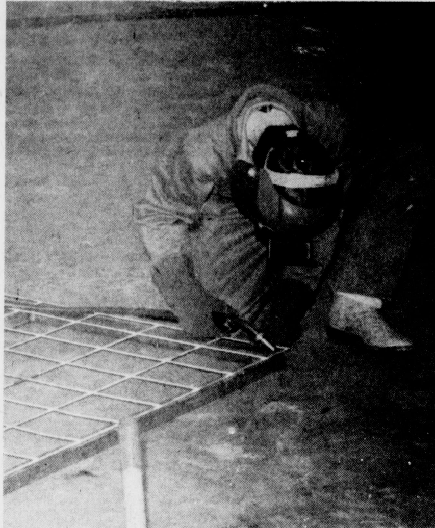
SEAN CLOSTI put skills learned in Rivercrest FFA to good use as he constructs a gate.
