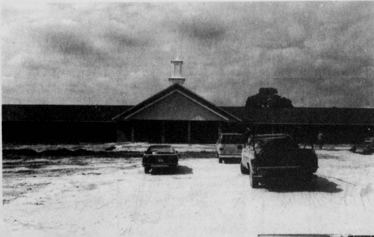
THE STEEPLE on the new Baptist Church now under construction in Bogata went up Thursday.
