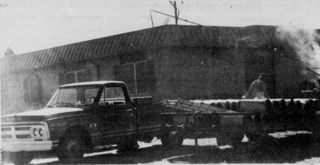
NEW ROOF-Red River Haven Nursing Home in Bogata is getting a complete new roof. The work is being done by Garcla Roofing Co. from south Texas. (Staff Photo by Mollie Williams)
