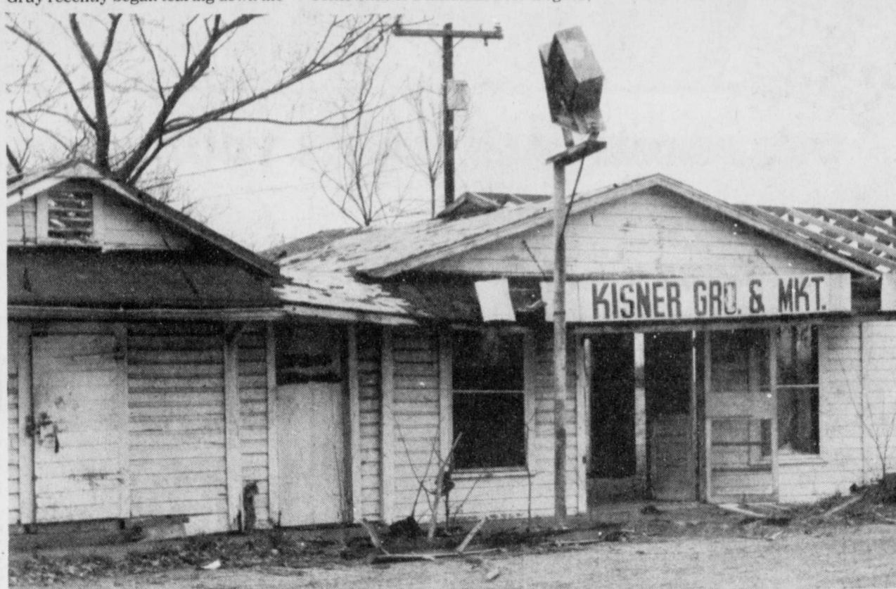
WORKERS began last week tearing down the building which was Kisner's Grocery Store. The
