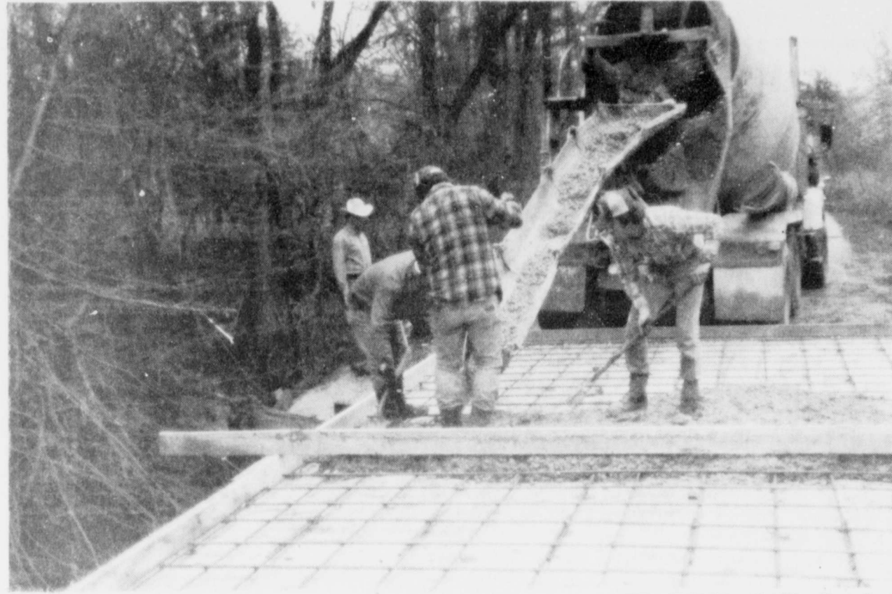
THE BRIDGE on the Pine Branch road is being replaced with a concrete one. County workers started the work last week. According to Precinct 1 County Commissioner, Druce Pirtle, the bridge should be finished this week. (Staff Photo)
