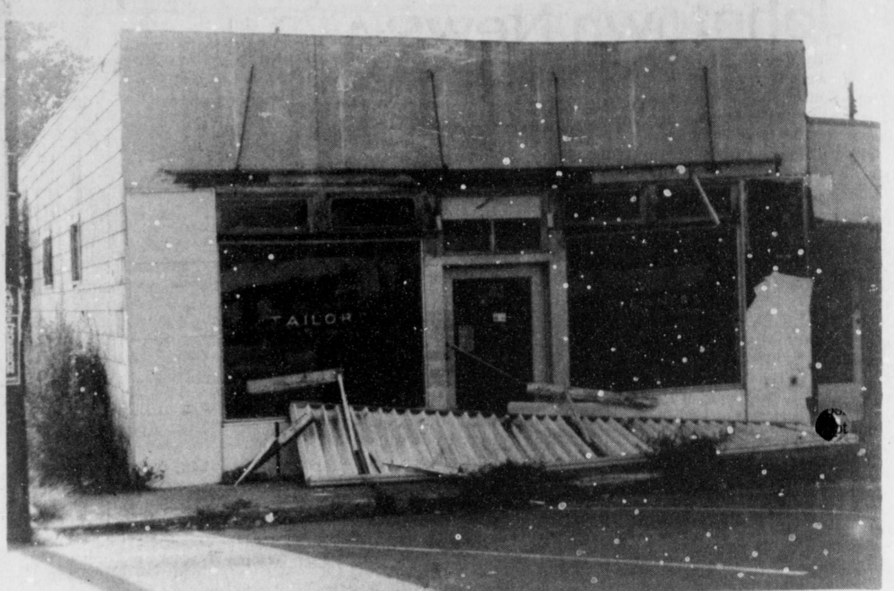
THE AWNING on the old Bogata Cleaners fell sometime over the weekend. The building dates back many years. (Staff Photo by Mollie Williams)
