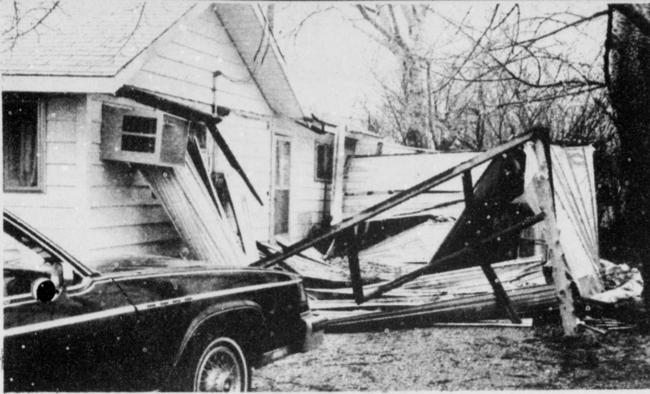
THE CARPORT at the home of Mr. and Mrs. Cliff Jones collapsed from the heavy load of hail that hit Talco Wednesday afternoon. (Staff Photo)
