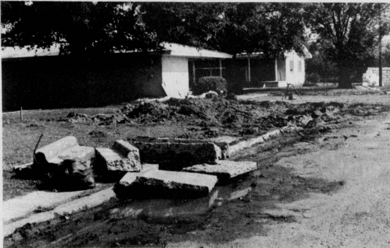
NEW LOOK-Workers are tearing out sidewalks to redo the walks and fix some off the street parking
