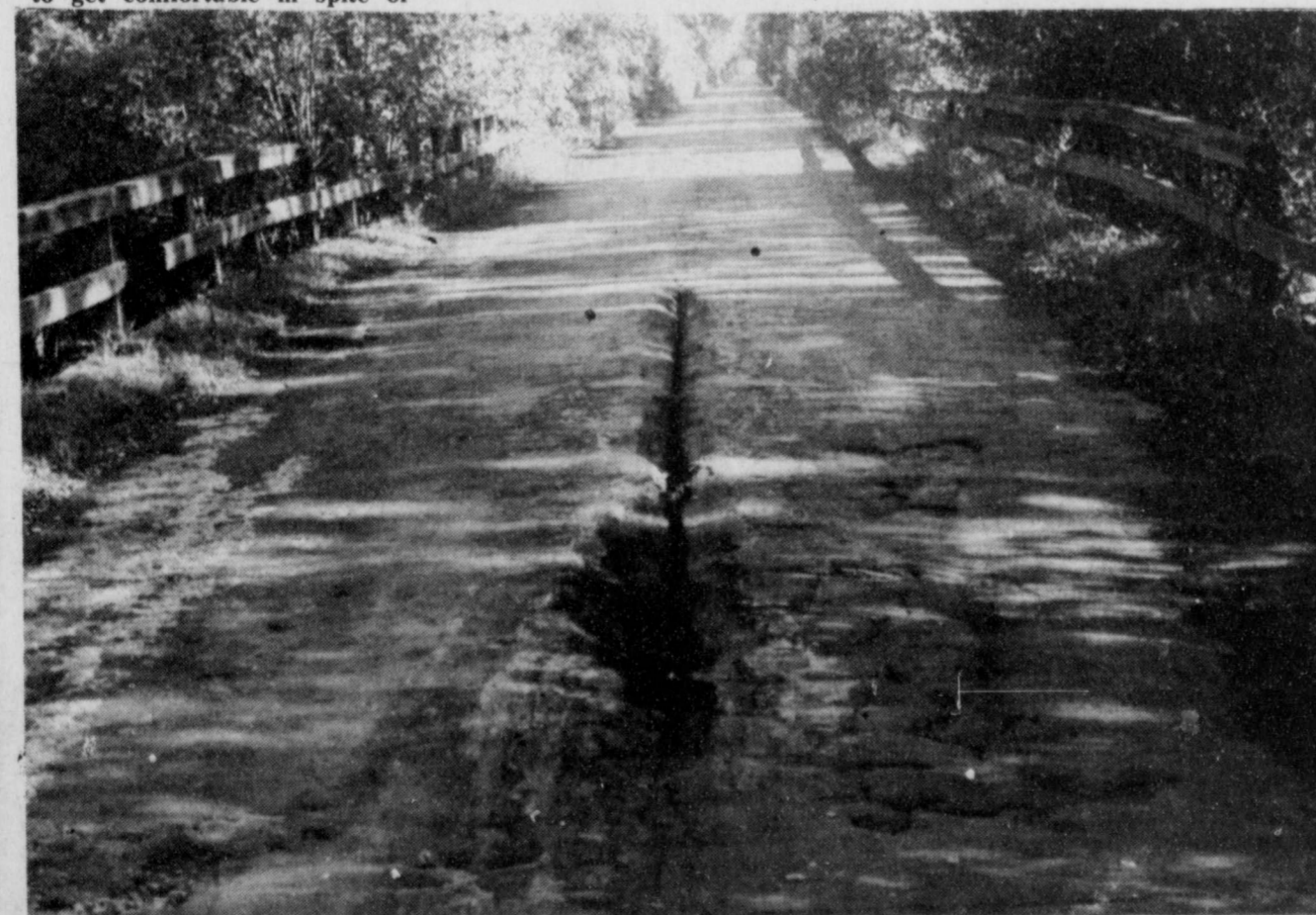
THE OLD BRIDGES that cross White Oak Creek between Meadow's Curve and Greenhill are to be replaced according to Titus County Commissioner.s The
