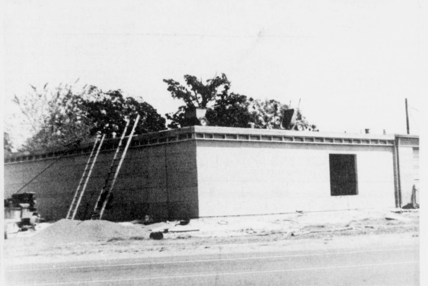
NEW ADITION-Bogata Elementary School has a new addition going up on the west end of the main classroom building. The additional space was much needed in the school. (Staff Photo by Diana Eudy)
