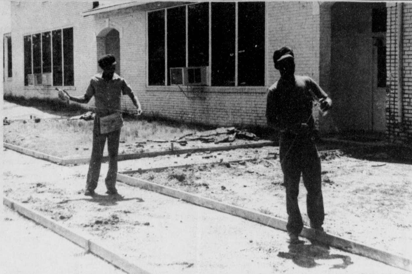
NEW WALKS—The Bogata Junior High building is getting new concrete sidewalks during the summer vacation. Walter Smith Jr. and Walter Smith lay the forms in preparation for the walkways. (Staff Photo by Diana Eudy)
