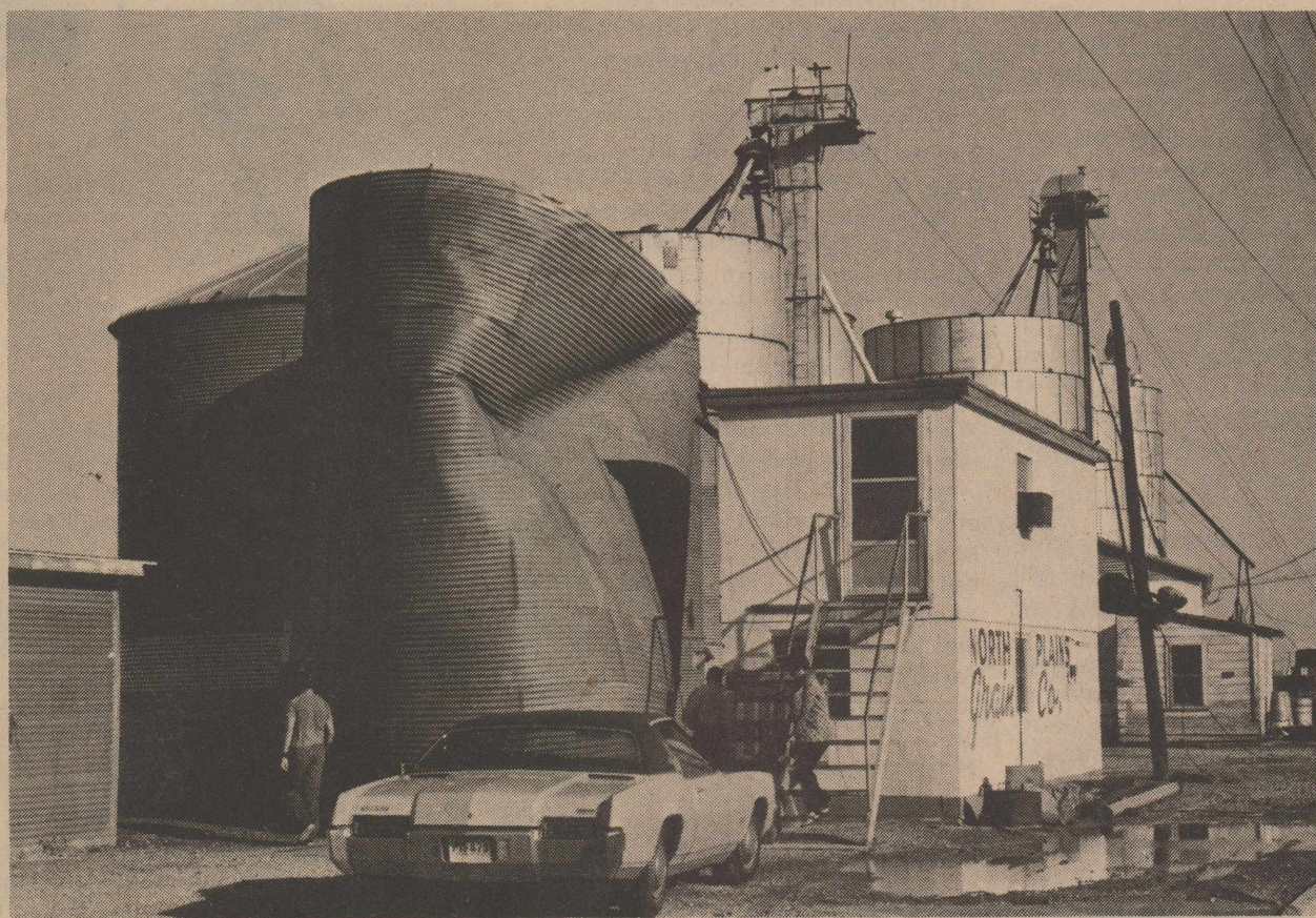
DAMAGE ON MONDAY MORNING --This huge grain storage tank was blown off its foundation at North Plains Grain Company alongside the Santa Fe Railroad in northwest Stratford during the storm Sunday night. The big tank had been blown into the office building but Manager Von Haggard said he had no estimate of dollar damage on Monday.
