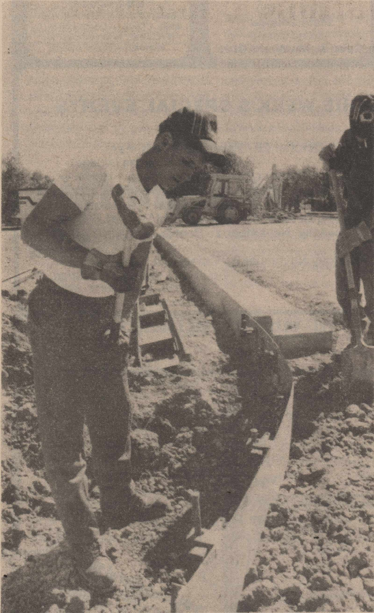
Airman First Class Robert Wanless, 64th Civil Engineering Squadron, sets the curbs for the new Reese Manor parking lot currently being constructed. (USAF Photo by SrA. Greg Spraggins)
