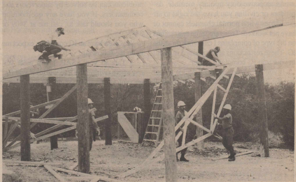
Members of the Reese Prime BEEF team deployed to Camp Rissington, San Antonio, Tx. to construct two new pavilions and renovate five hardback tents, along with various other safety related projects they accomplished to help add comfort and aesthetics to the camp. (USAF Photo)
