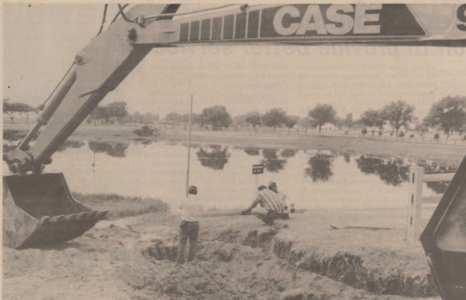
The 64th Civil Engineering Squadron's Carpenter, Equipment, and Sheet Metal Shops began excavating an existing ditchline Aug. 29 to install a 30-inch culvert pipe, headwalls and junction box to help improve drainage and eliminate flooding of the Base Picnic Area. The work is scheduled for completion next week after over 500 manhours of work and an estimated cost of $13,875. Shown is (left to right) Mr. James Cox, Mr. LeRoy Robertson and Mr. Jesus Martinez.
