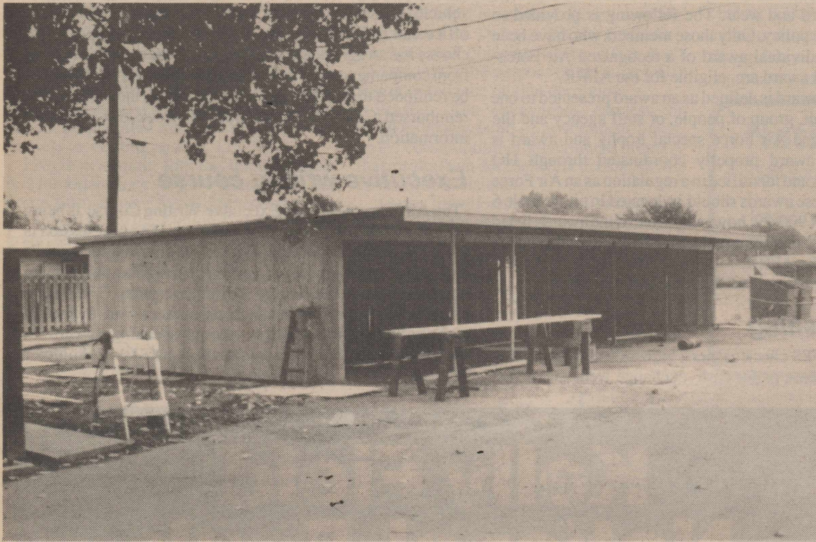
The 64th Civil Engineering Squadron Carpenter Shop has recently finished another major construction job by completely rebuilding the burned out carport on the 800 block of Mitchell Blvd. in Reese Village. SSgt. David Manchester, NCOIC of the shop, SrA. Terry Carpenter, A1C Wallace Greene, Mr. Richard Higgins and Mr. John Apodaca. The 1500 square foot structure required approximately 380 manhours at an estimated cost of $14,000. (USAF photo)
