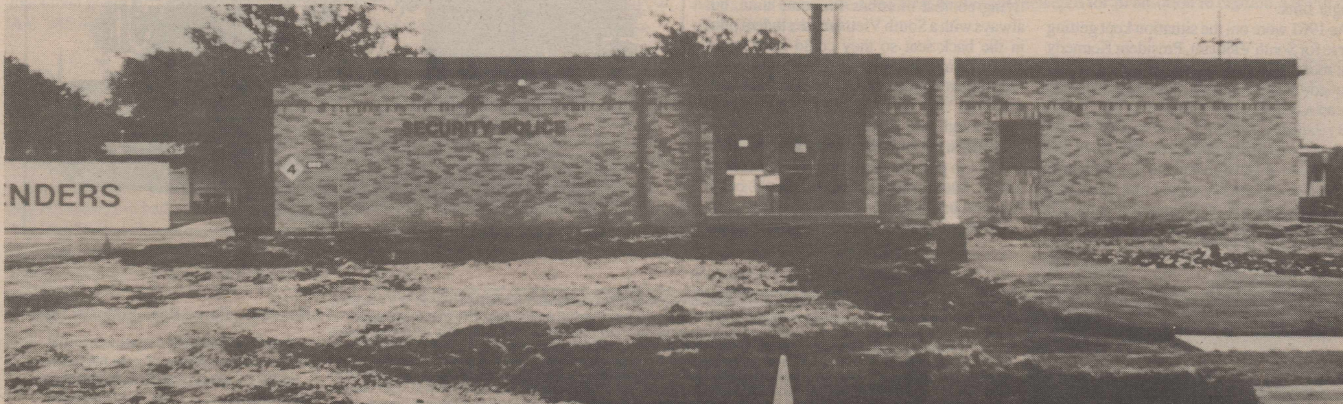
Earthquake? No, but the Security Police building will become larger and better as all SP functions are consolidated into the same complex. (USAF photo)
