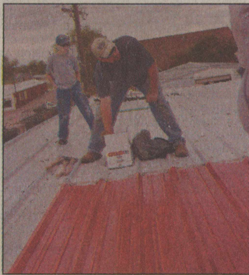
The crew securing the metal sheets in place with the special screws to prevent future damages.
