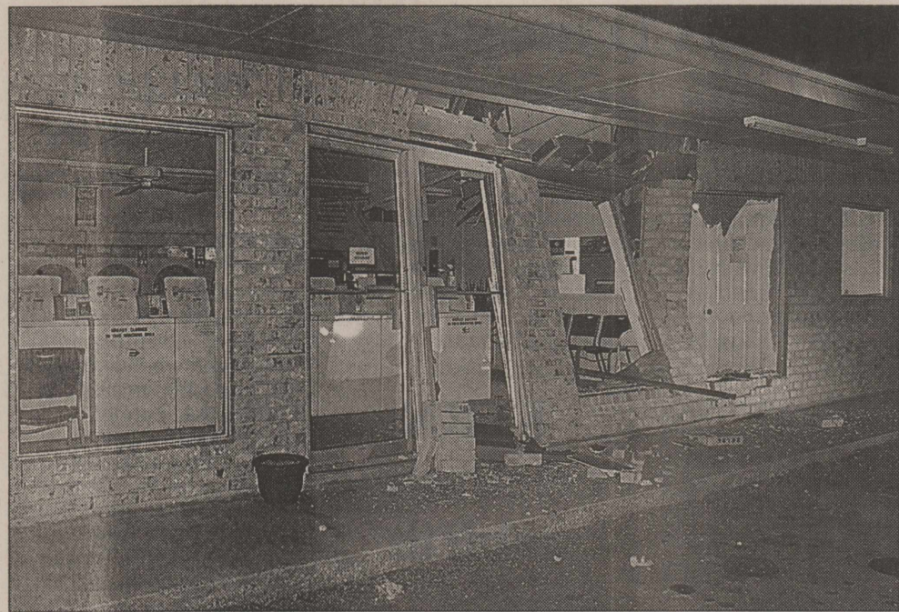
PHOTO: CONTRIBUTED The front of the building suffered extensive damages after the wreck occurring on Tuesday, October 4, 2011.
