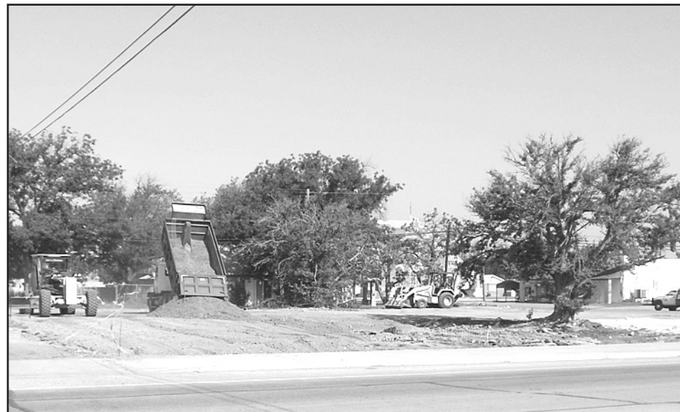
DIRT WORK —The City of Haskell and Haskell County employees began work on the parking lot located just north of Haskell County Insurance Co. on Thurs., Aug. 1.
