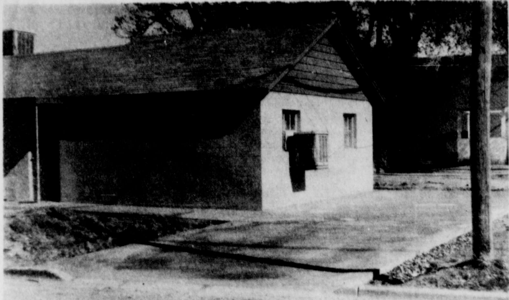
ABERNATHY POLICE DEPARTMENT gets a new concrete drive and sidewalk, which were poured last week. Improvements are almost complete at the police station as the inside has been remodeled and the outside repaired. (Review Photo)
