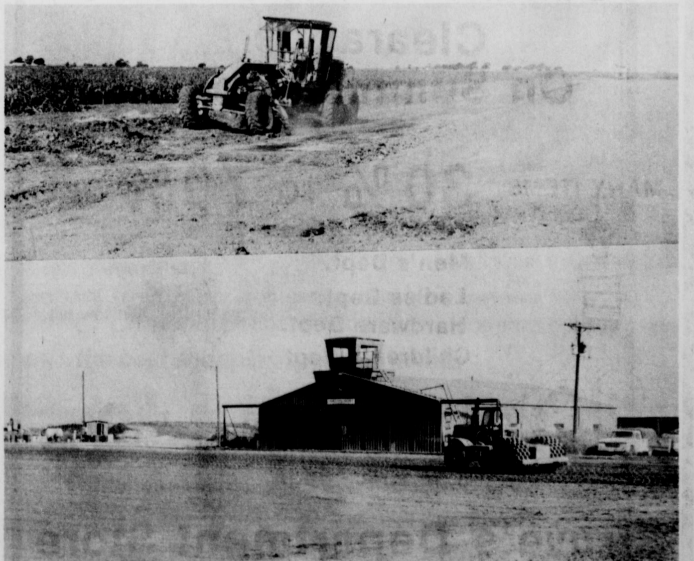
AIRPORT IMPROVEMENTS taking place at the Abernathy Airport. Pictured are graders smoothing and packing the soil base on the taxi-way strip. The old asphalt air strip, which was constructed in the 40's, is being completely removed and will be replaced with a new base. (Review Photo)
