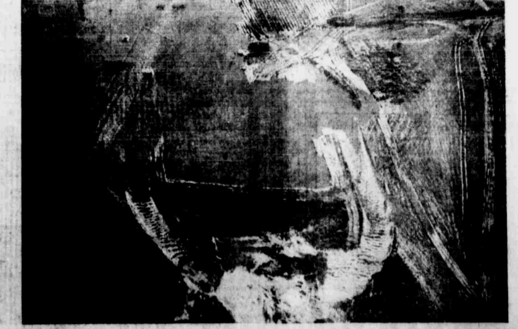
A TEMPORARY DAM at Millers Creek was completed shortly before recent rains completely halted construction. Water backed up behind the dam will be used to pack dirt for the permanent dam. According to J. H. Strain, contractor, the rains which stopped construction for over a week will help later when water is needed for the packing of the permanent dam. According to Mr. Strain, "There was not an adequate supply of water nearby and we would have had to haul water. The supply now on hand will save much time and effort later." (Staff Photo)
